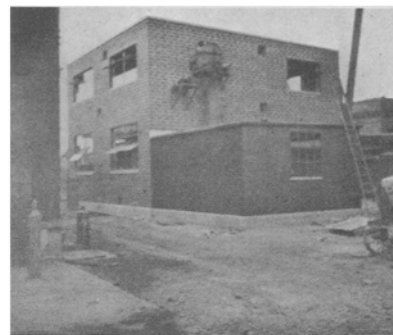
Extraction Plant Building Under Construction. The One-Story Section Is Used for Storing Spent Bleaching Materials as They Are Brought Over from the Refinery.
